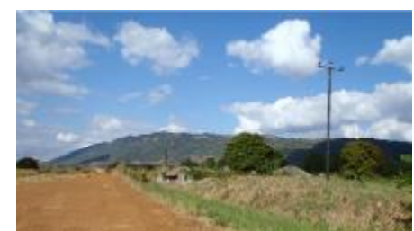
Power Lines near Balama
